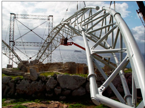
Fig. 1. Archaeological shelter at Hagar Qim (design by FormTL, photo by M. Ansaloni): a – view; b – installation; c – frame during installation.
